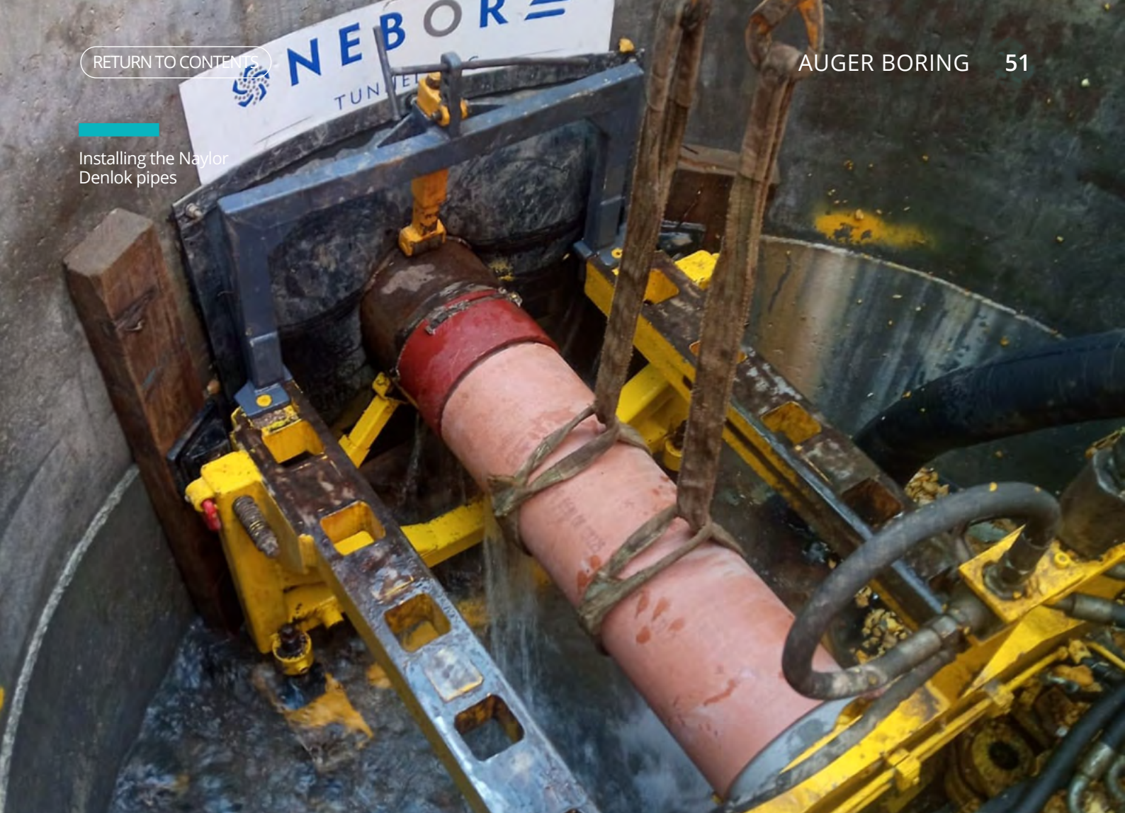
The rubber gate used to control water ingress during the bore launch cycle
